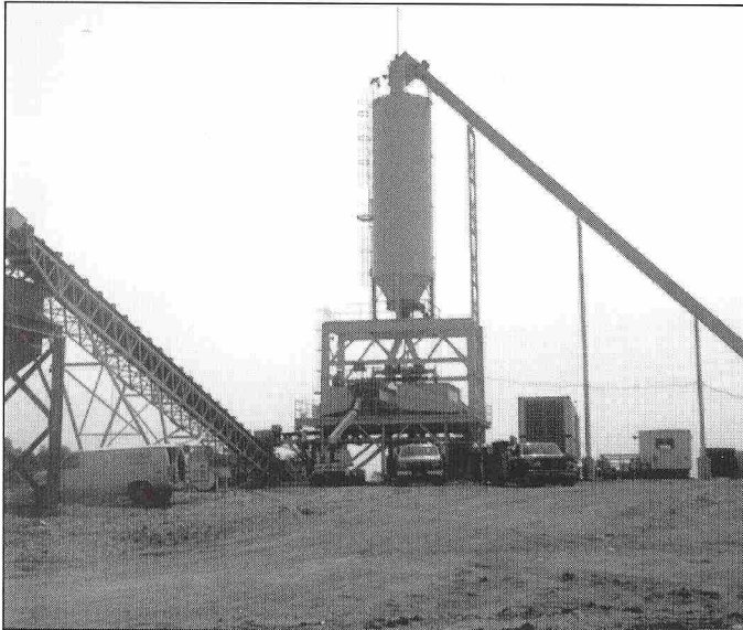
Cement kiln dust mixed with harbor dredged mud will fill a 60 acre parking lot with as much as six feet of fill.
