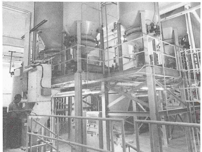
The sophisticated materials handling system at Tremco includes Bin Activators to assure positive discharge of stored materials.
