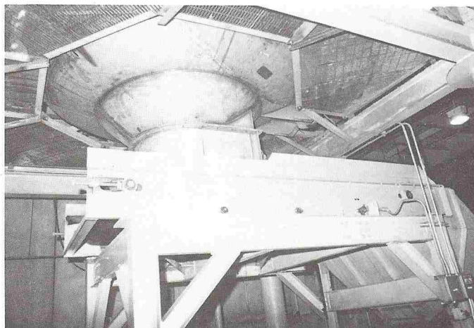
Operating in conjunction with the Bin Activator at Georgia-Pacific is a volumetric Heavy Duty Belt Feeder which provides the capability to regulate downstream flow so that it "locks in step" with input into storage from the chip stockpile.
