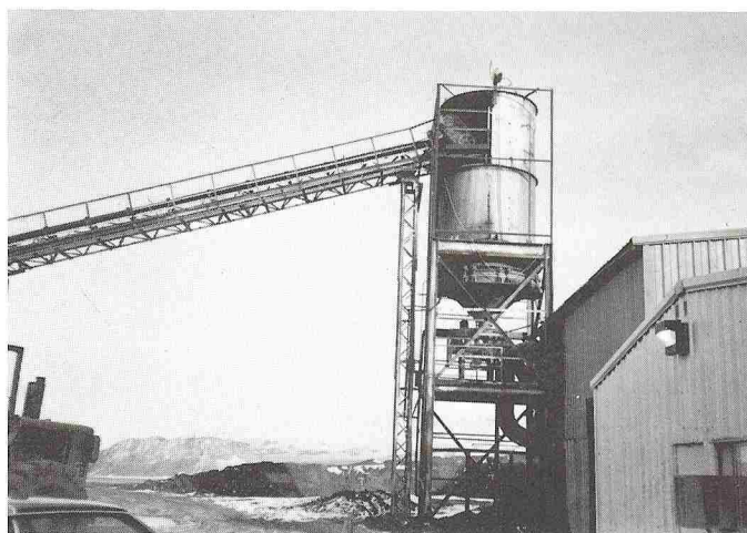
IMCO Services moves their barite mixture by belt conveyor to a cylindrical storage bin where the Vibra Screw Bin Activator discharges it with a dependable and consistent flow.
