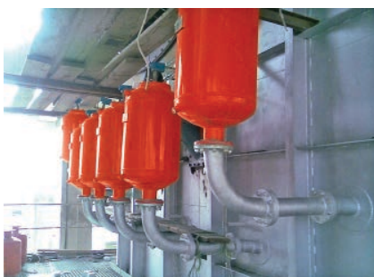
FIGURE 8. Silo air blasters are effective at dislodging immobilized materials in storage bins
